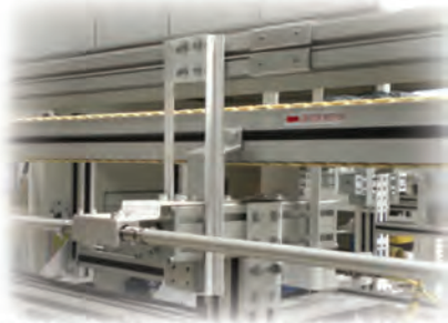
Automated side guide installed at straight section
