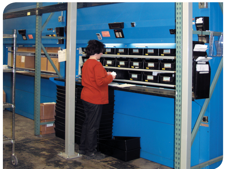
Two vertical carousels located between mezzanine supports are used for packing and redressing.
